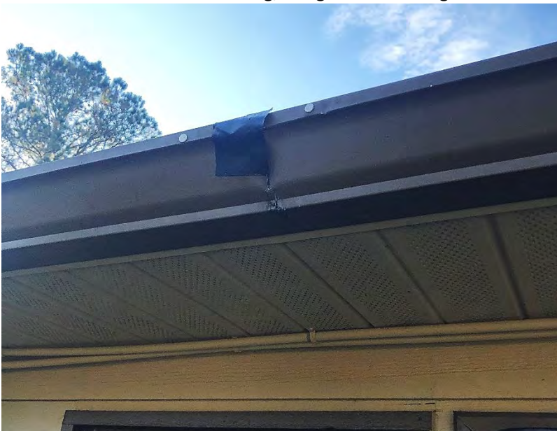
Figure 5 - Gutter Seam Building 1
