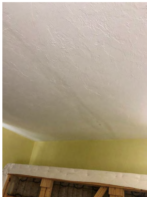
Figure 1 - Ceiling Stain Unit 102
