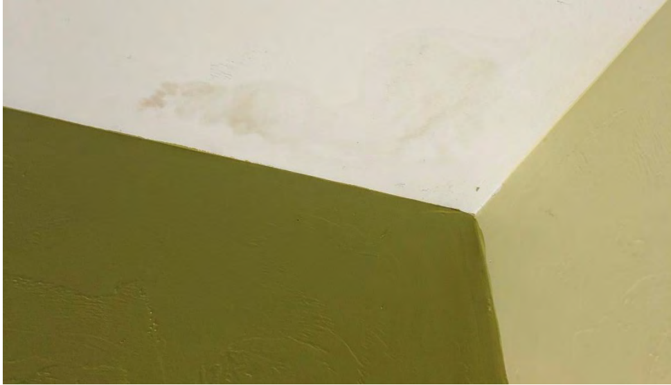
Figure 2 - Ceiling Stain Unit 103
