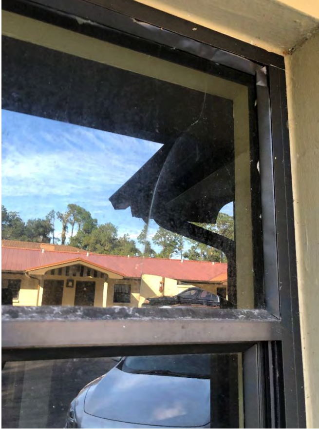
Figure 11 - Broken Window Unit 118
